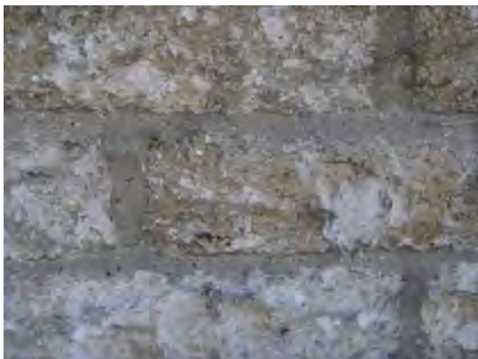
Malton Oolite stonework beneath Hildenley limestone cornice (which will date from early C18 and have been raised with the building). Note remnants of copperas pigment to both cornice (above) and coursed rubble. Opc mortar.
