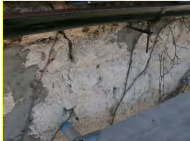
South and east elevations of the addition, showing serious decay to oolite of east wall; opc render to south.
