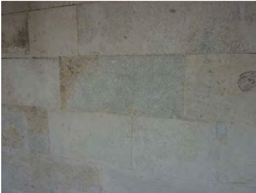
Reasonably colour matched but cementitious render repairs to oolite blocks, 2 nd floor, now loose.
