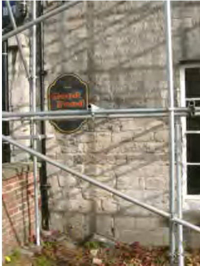
trial panel of moderately sulphated stonework, June 2010. Uncleaned masonry above and around signage.
