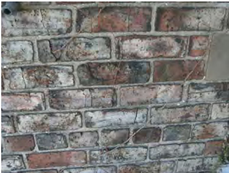
Brickwork of C19 addition to east of above and to west of east range. Original lime pointing a little eroded back but sound.
